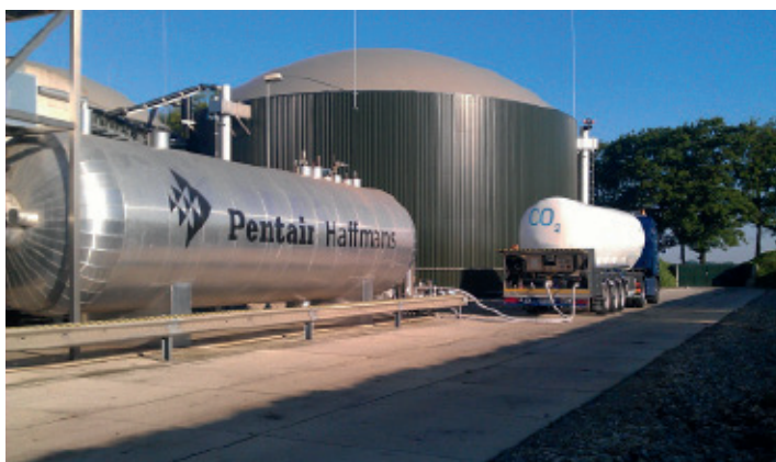
Biogas plant and CO 2 buffer tank
