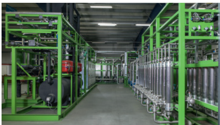
Turnkey biogas upgrading system
