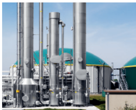
Biomethane plant Semd - Germany
