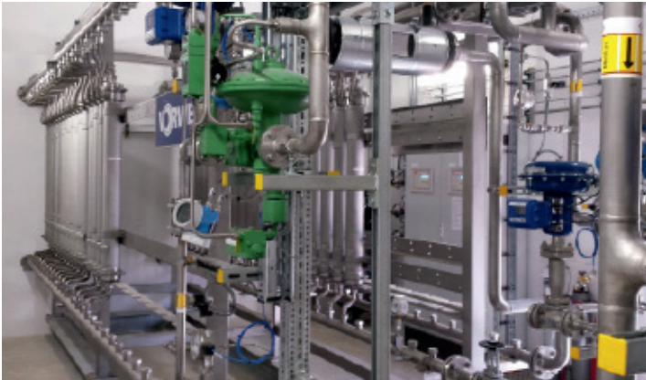
Indoor installation of membranes for CO 2 separation
